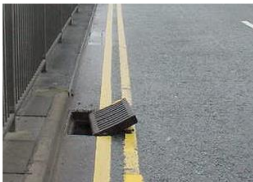
Displaced gully grate
