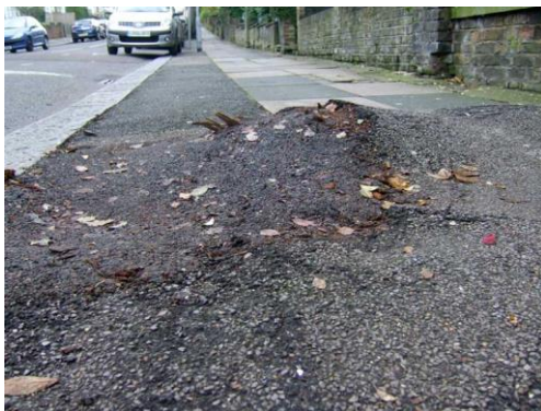
Tree route damage to footway
