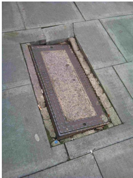
Rocking inspection cover
