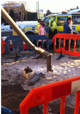
Damaged in RTA
