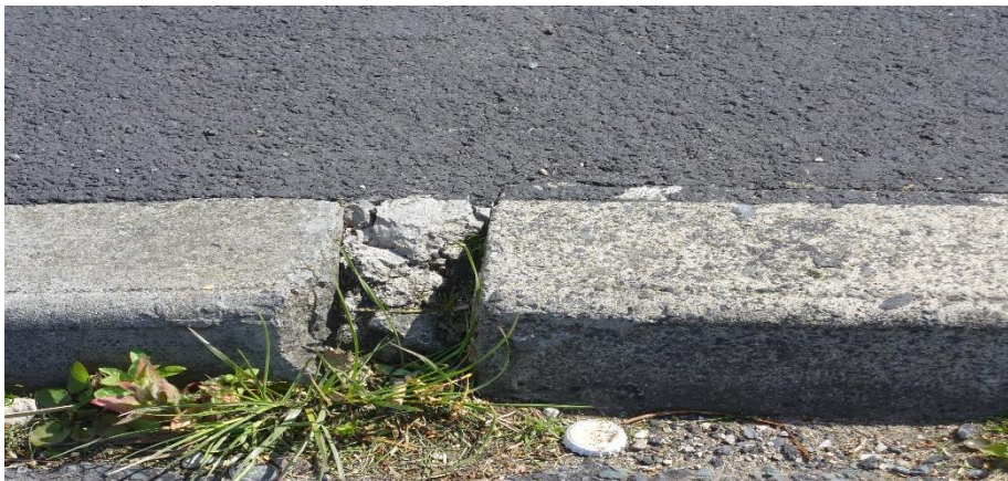
Gap between kerbs
