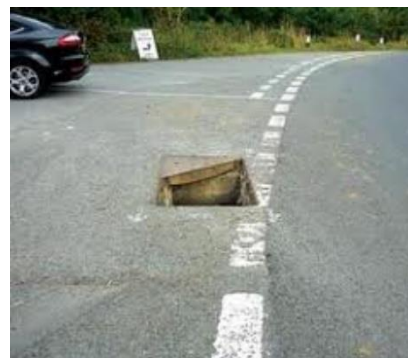
Missing Inspection cover
