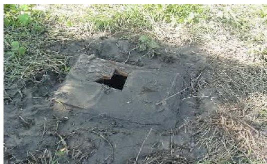
Broken Inspection cover
