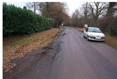
Depression and heave along edge of road
