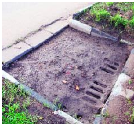
Gullies blocked by silt
