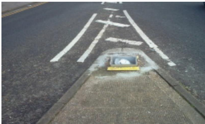
Missing keep left bollard
