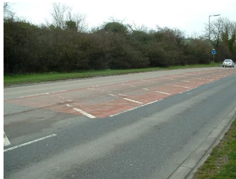
Loose material in centre of road
