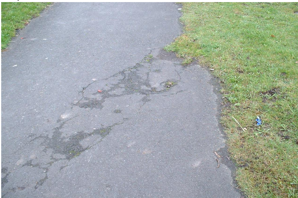
Subsidence in footway
