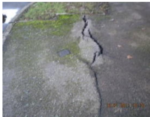
Tree route damage to footway
