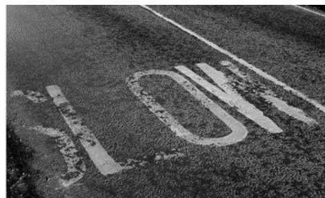
Approx 30% faded markings
