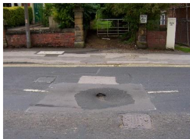
Depression in centre of road
